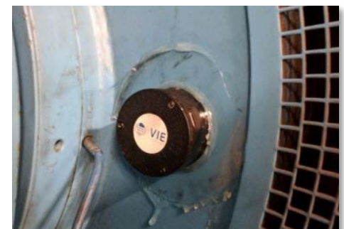
OPA sensor installation
