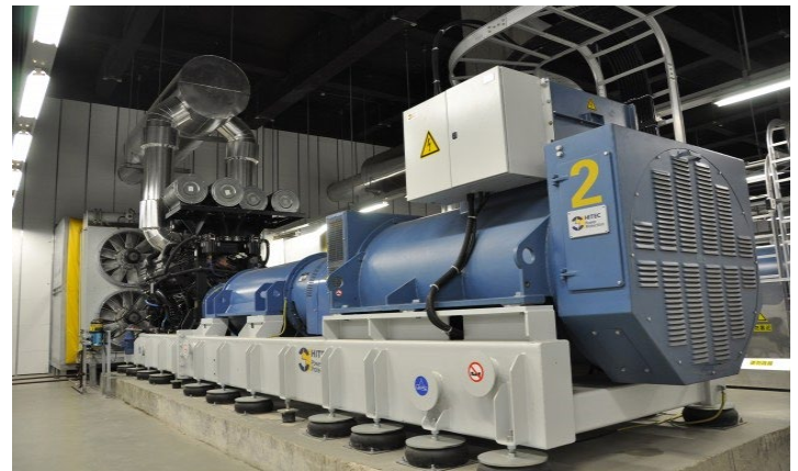
HITECH Rotary UPS
